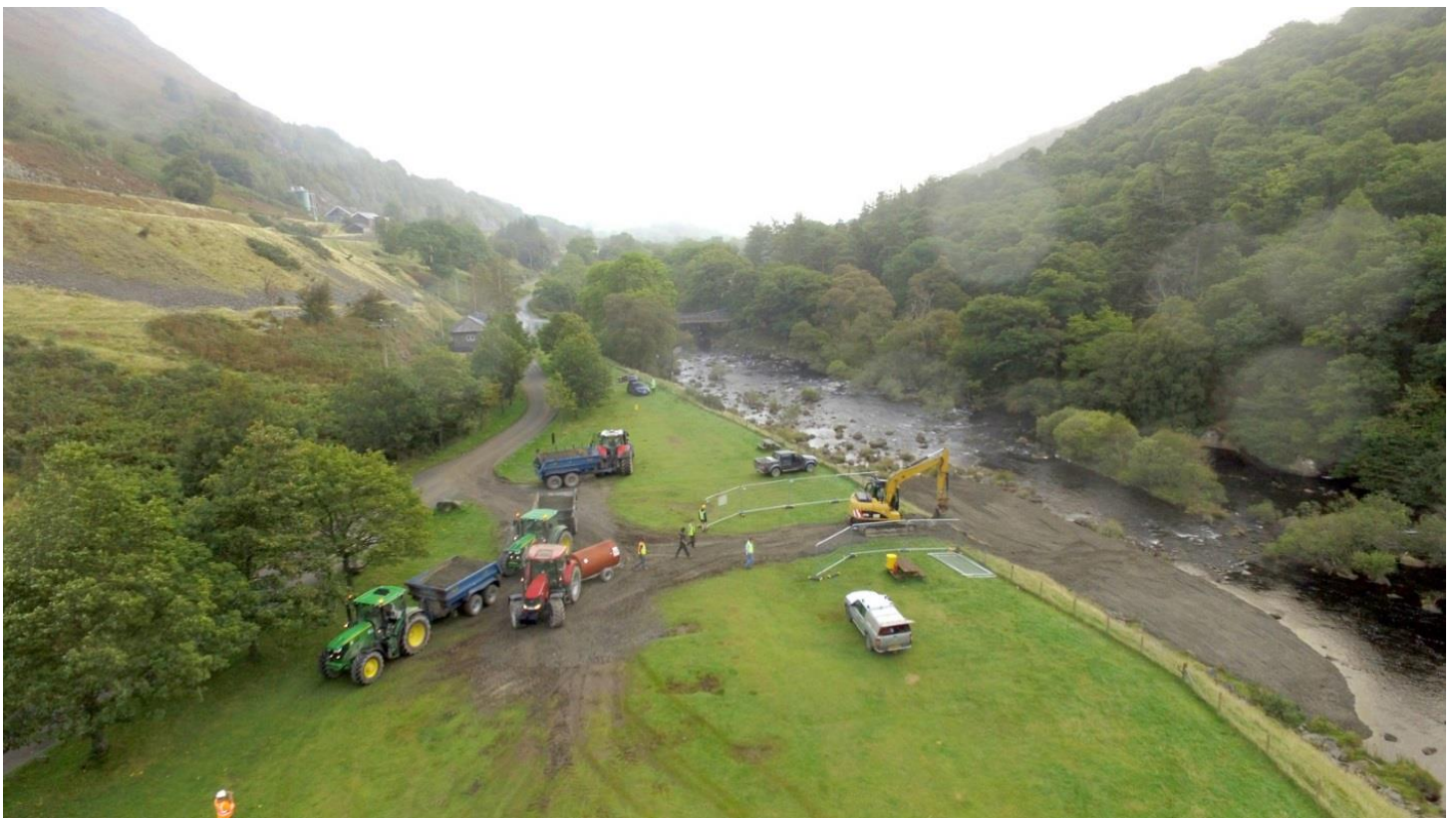
Figure 8: At Site 4 a platform was created with the first loads of gravel from which the remaining loads could be placed into the river channel
