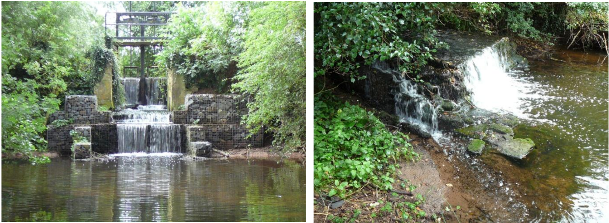
Figure 43&44: Barriers to fish migration identified during the walk-over survey
